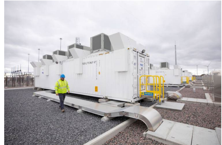
Scale: 1 megawatt of storage is the physical size of a shipping container
